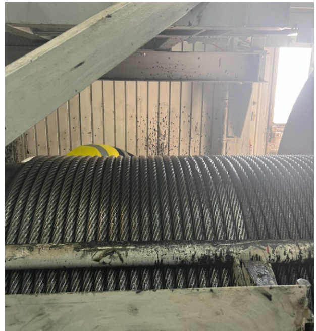
FIG 3 – Visually you can see the left-hand side of the drum has cleaned and re-lubricated wire rope vs the right-hand side drum rope which has yet to pass through the cleaner and Viper WRL.
