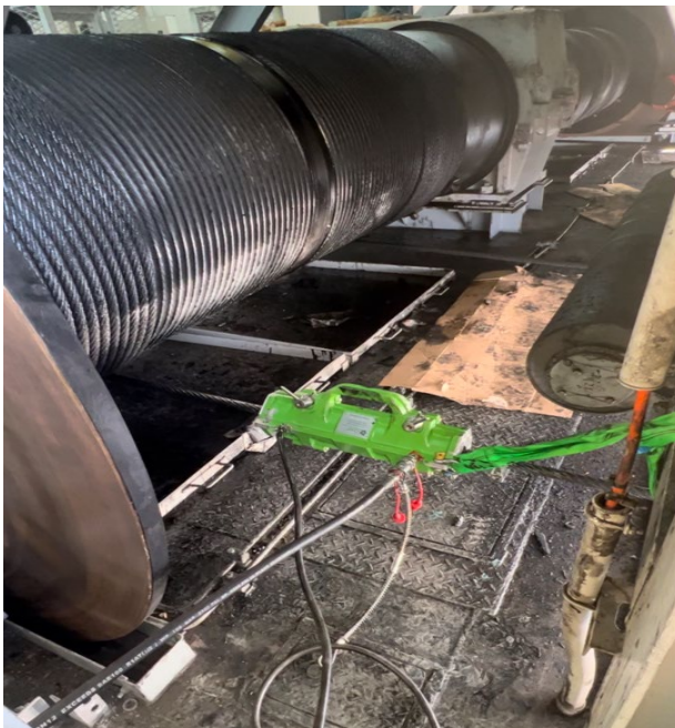
FIG 2 – Viper WRL Mid is set up in the drum wire room, cleaning and applying new Viper Wire Coating Grease whilst rope is feeding back onto the drum.
